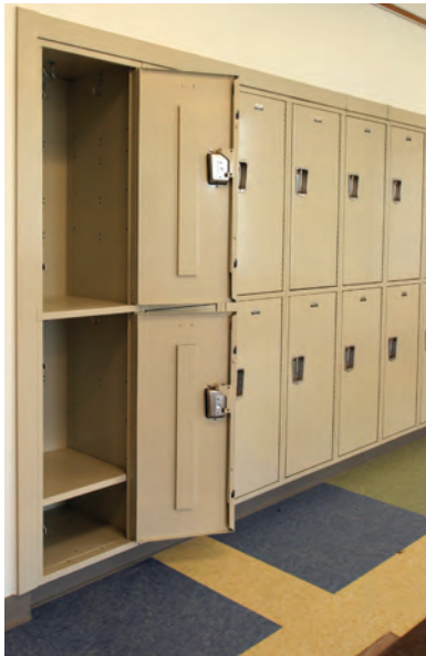
ADA locker has shelf at least 15 inches from floor.
