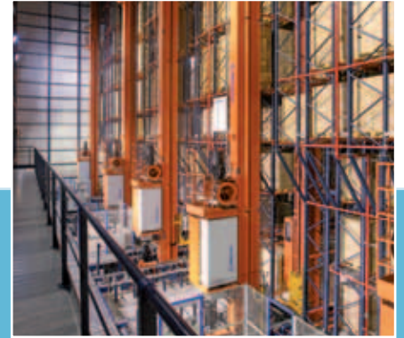
Single-mast and double-mast automatic stacker cranes
